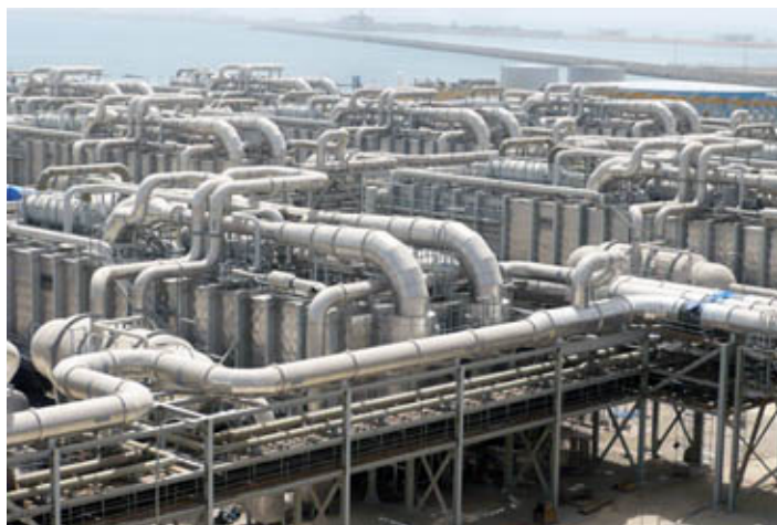
Marafiq MEDs with Steam and Vapor Ducting
